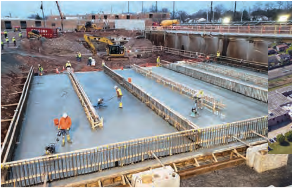
Construction is well underway as workers pour the base slab of the ozone contactors.
