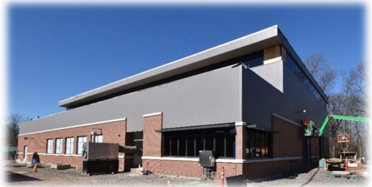
The Park Avenue Treatment Plant is delivering water in compliance with state and federal standards.
